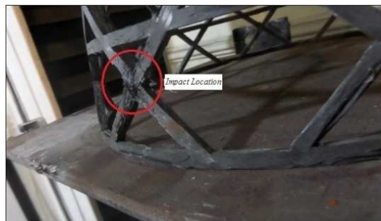
Fig. 11. The impact location on the structure and the damage done.
